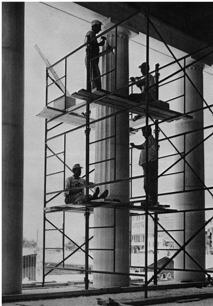
22. FLUTING A DORIC COLUMN. In keeping with ancient practice the lower front columns, each consisting of three drums and a capital, were channeled after erection. In this way the lines could be carried through with complete precision. Here, as commonly in the Hellenistic period, the lower third of the shaft was left unchanneled and so was less subject to damage from traffic.
