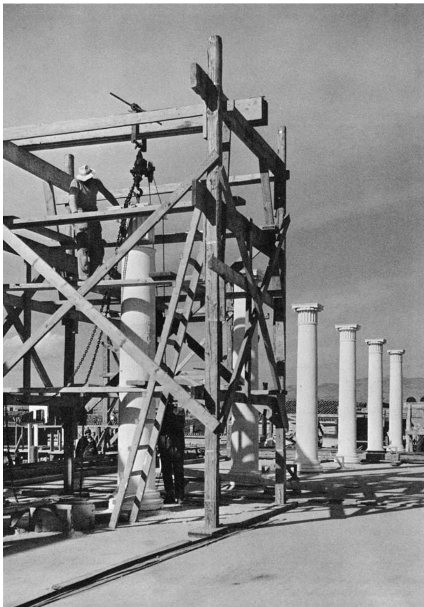
23. ERECTING THE INNER COLUMNS OF THE UPPER FLOOR. Cuttings in the ancient blocks indicate that the original builders, like the modern, had hoisted the heavy members by means of block and tackle. The inner columns of both storeys were left smooth since fluting is ineffective unless the sun can strike across the column.
