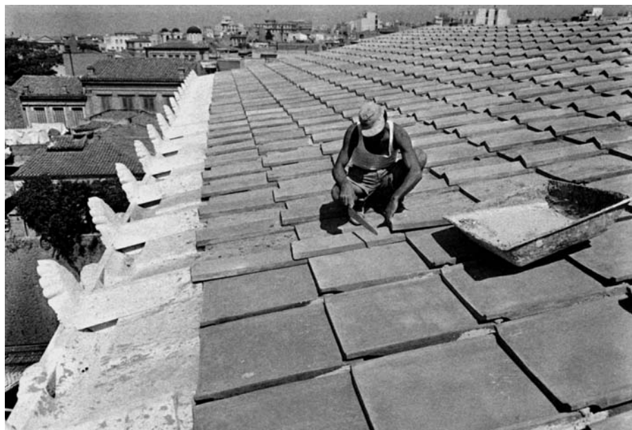
20. ROOFING. The eaves tiles above the façade were of marble, the rest of terracotta. The design was recovered from fragments found on the site, and the new tiles were made to order in Piraeus.
