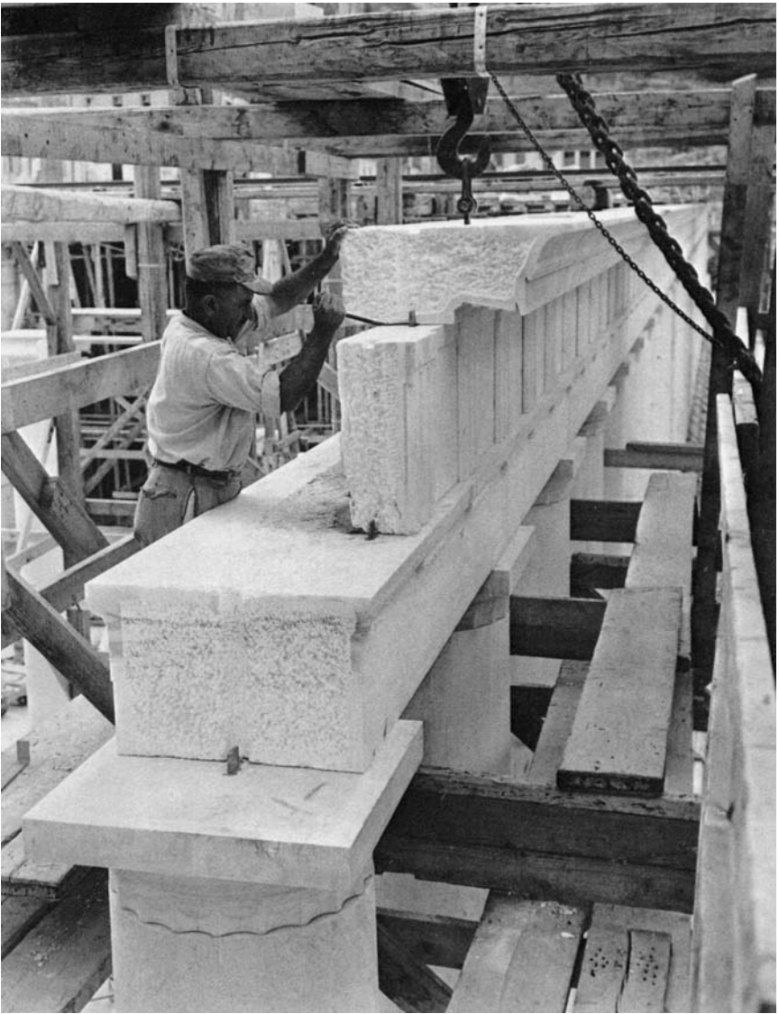
24. ASSEMBLING THE DORIC ENTABLATURE IN THE LOWER STOREY OF THE FAÇADE. Above the capitals comes the massive lintel or architrave, then the Doric frieze of triglyphs and metopes, and finally the cornice. The blocks were secured to one another by means of metal dowels.
