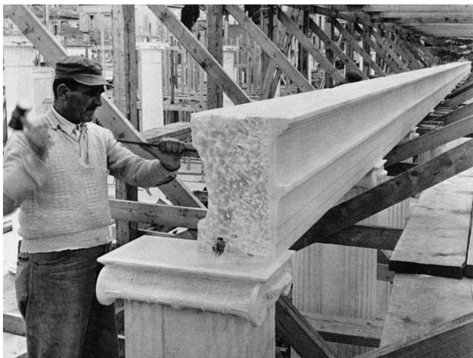
25. THE IONIC ENTABLATURE IN THE FAÇADE OF THE UPPER STOREY. Architrave and frieze are here combined in a single member which will support the upper cornice and the eaves of the roof.
